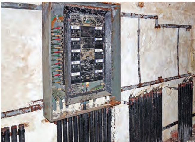
Zeppelin/Ranet - comms cables and switching gear. Photo Vin Stenhouse
